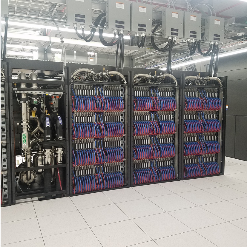
Figure 10: Frontier (with the doors off) has 3 computer cabinets for every cooling unit (CDU)
