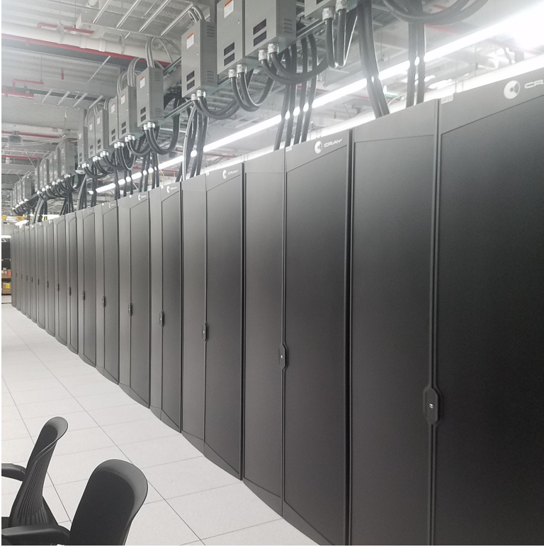
Figure 9: Frontier's Front 12 cabinets
