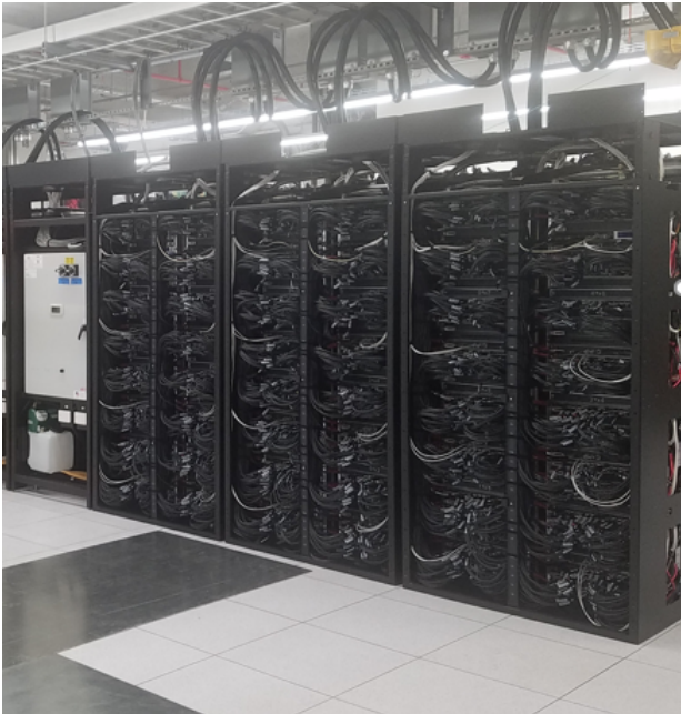
Figure 11: Rear View with Doors Off; Rear of cabinet has power and all the interconnect wiring.
