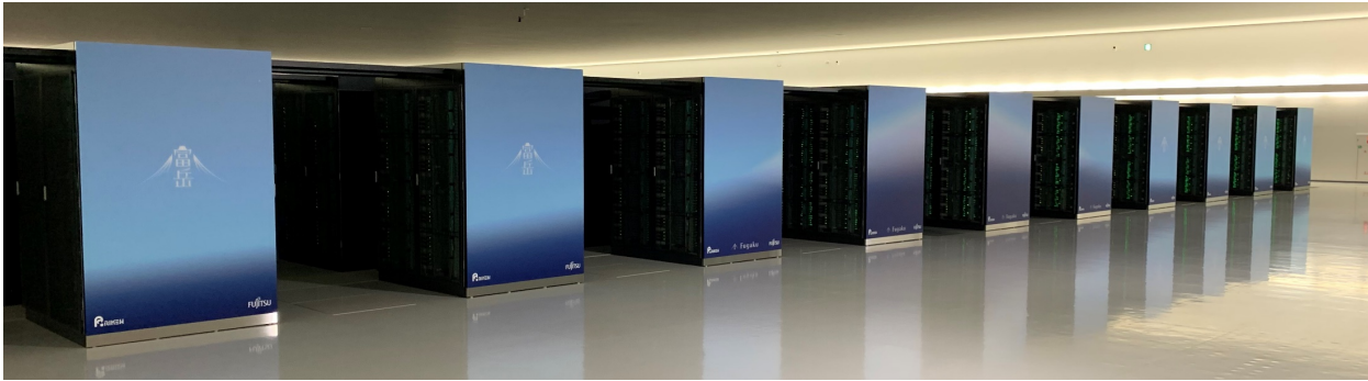
Figure 1. Fugaku System as installed in RIKEN R-CCS
