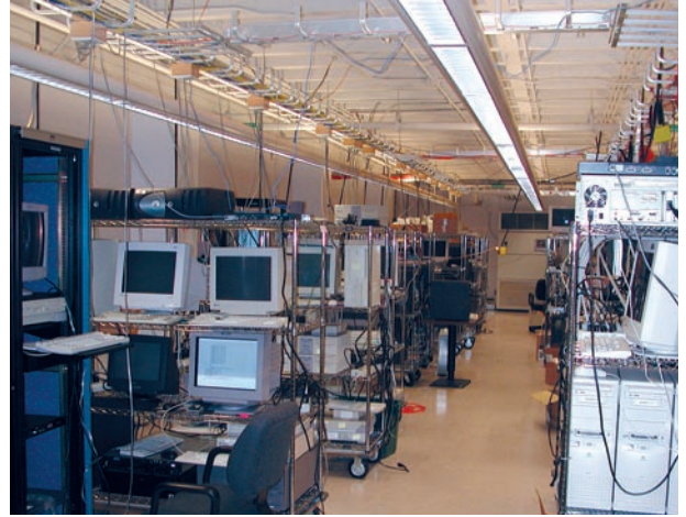
State-of-the-art machine room
